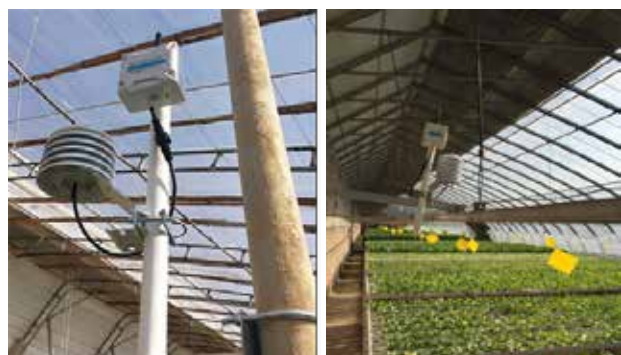
• Above (left) Monitoring Sensor (installed in Agric greenhouse-right)
