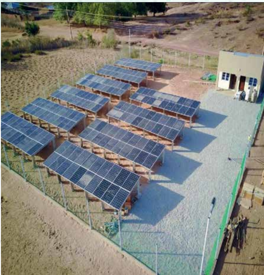
NEWMAP/Nigeria Green Bond Financed Mini Grid in Torankawa, Sokoto State
