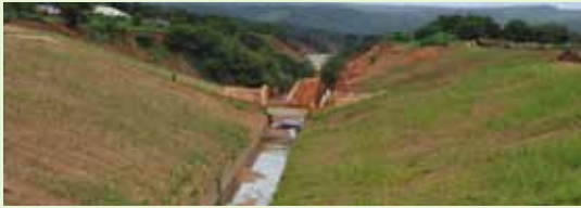
A well terminated drain with bio-remediation work in Auchu, Edo State.
