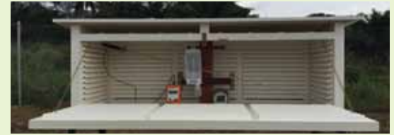
Automated weather system installed in Imo State.
