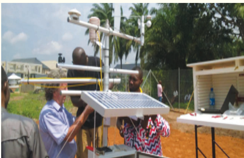
Installed Automatic weather station (AWS) in FUTO Owerri
