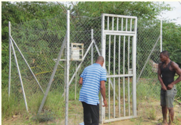
Installed automatic hydrological station in the AIRBDA
